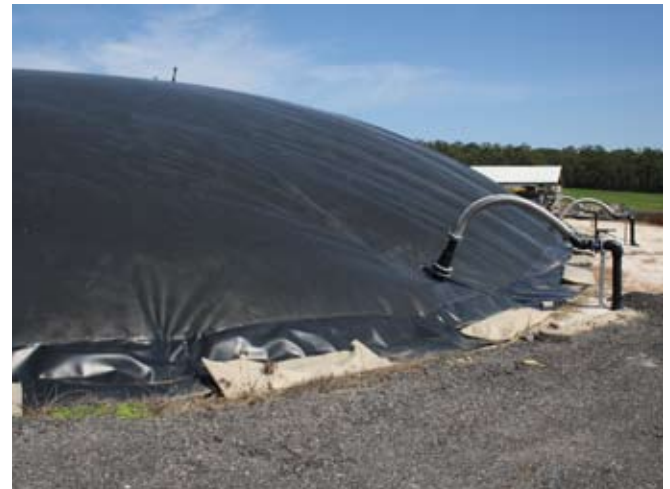
Figure 4: Anaerobic pond cover in place, with gas collection pipes
